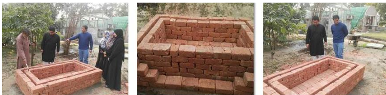
Figure 1: Zero-energy cool chamber (ZECC) construction at the Institute of Agricultural Sciences University of the Punjab, Lahore.
